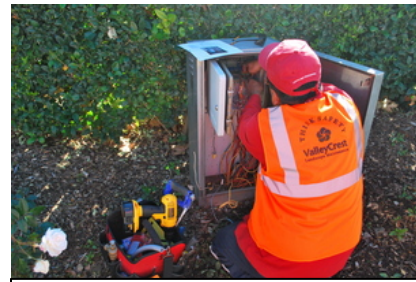
SMART CONTROLLERS ADJUST YOUR IRRIGATION SCHEDULE BASED ON DAILY WEATHER CONDITIONS. CONTROLLERS TYPICALLY GENERATE ANNUAL WATER SAVINGS OF 15-20% AND A RETURN ON YOUR INVESTMENT IN 2-3 YEARS.
