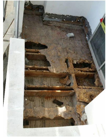
INVASIVE REPAIRS DUE TO LACK OF MAINTENANCE
